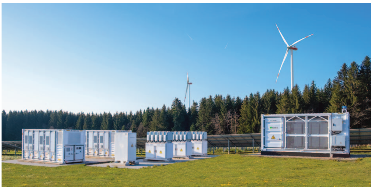
Spitalhöfe solar park, 7 MW PV coupled with 3 MW / 4 MWh BESS. Pfaffenweiler, Germany.
