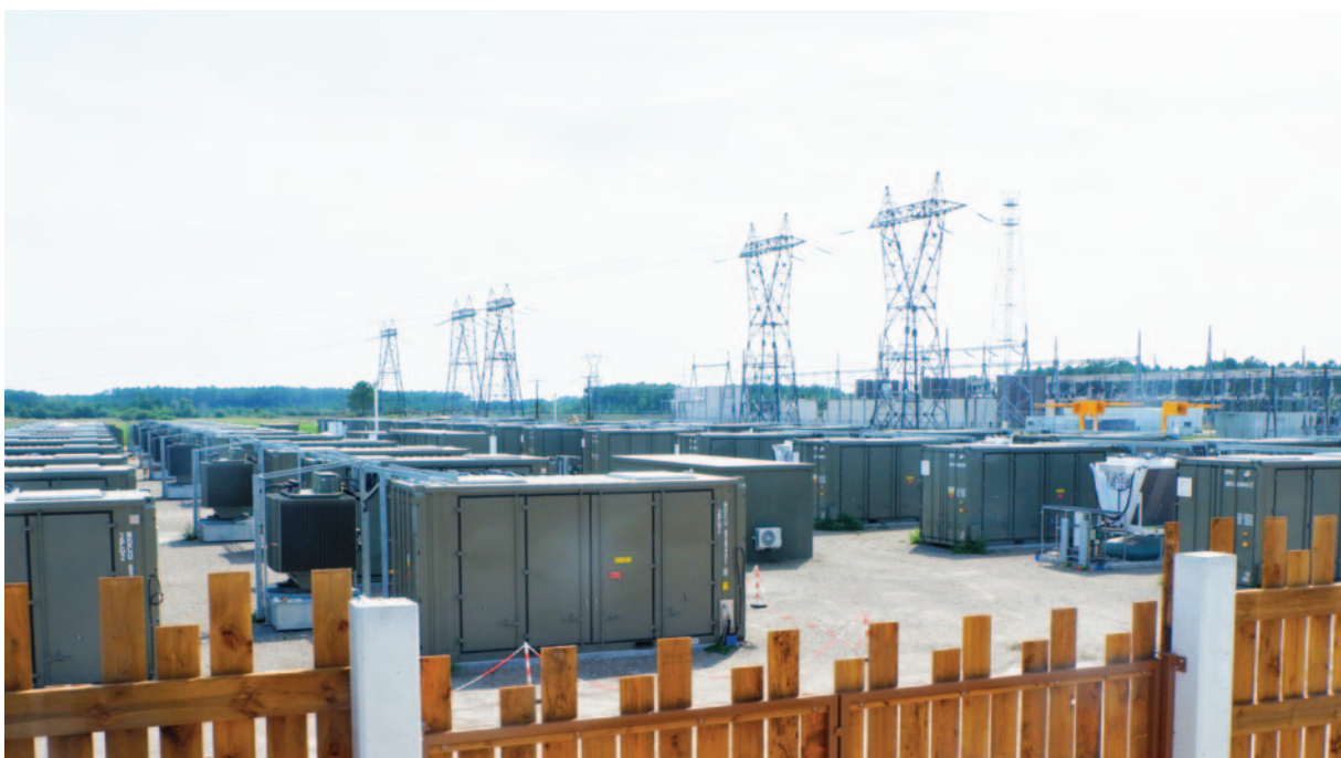
Claudia storage project, 105 MW BESS. Saucats, France.
