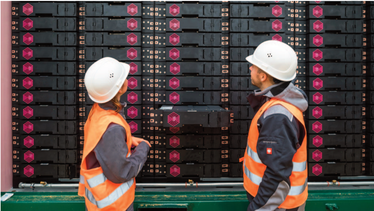
Deisenhausen solar park, 18.2 MW PV coupled with 6.2 MW / 20.7 MWh BESS. Krumbach, Germany.
